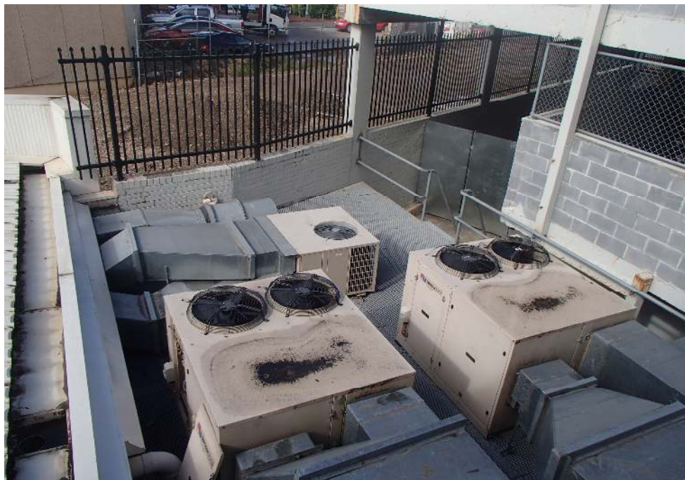
Photograph 10 (2016) - Looking at Air Conditioning Units Located in the Middle (eastern) Section of the Site
